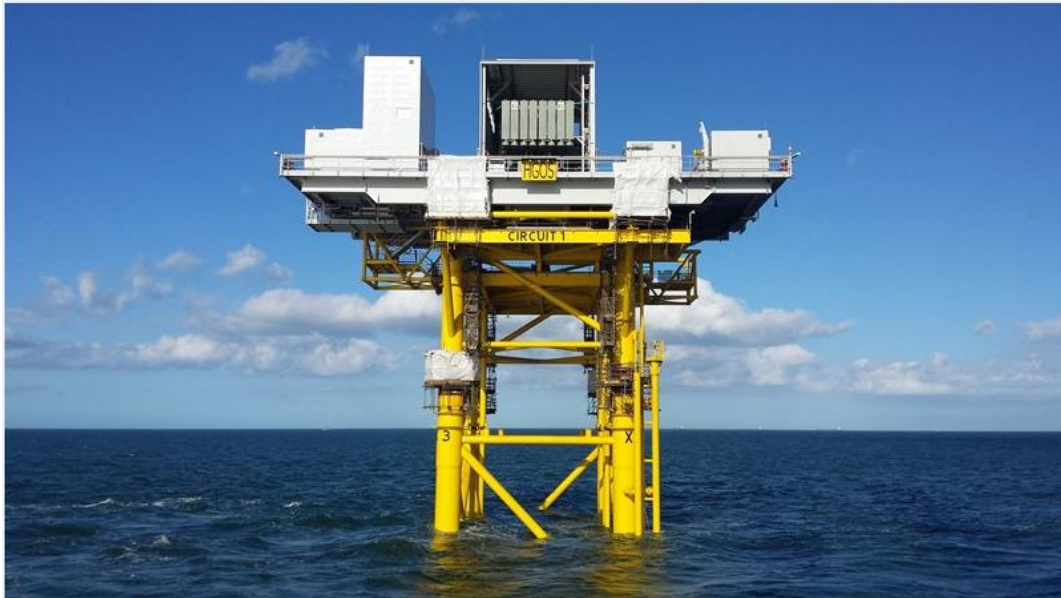
Figure 4-4. Example of a typical installed OSP.
