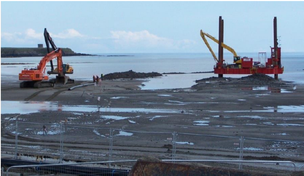
Illustration 4.20: Open cut trenching beach excavations – tracked excavators and barge-mounted excavators (Source ETA Ltd)
