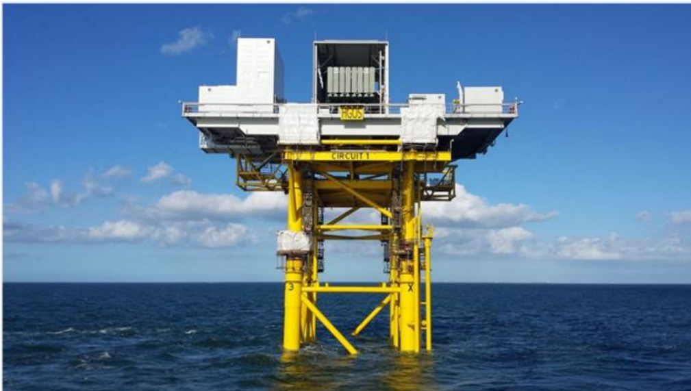
Illustration 4.15: Installed substation (Pictures courtesy of CG. Copyright ®vanoordbv-mennomulder.com)
